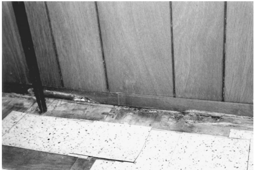
Fig. 10-4. Rotting and delaminating section of raised wood floor in finished basement. Condition is caused by constant wetting from water seepage into the basement.
