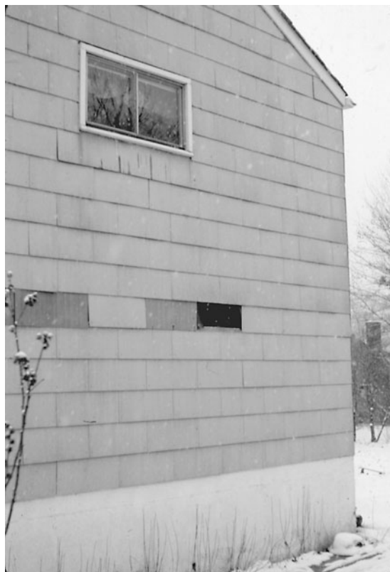
Fig. 5-4. Missing and patched (mismatched) asbestos-cement shingles.
