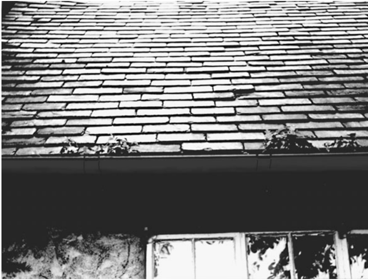
Fig. 3-12. Gutters must be cleaned periodically to be effective. Note the weeds growing out of this gutter.
