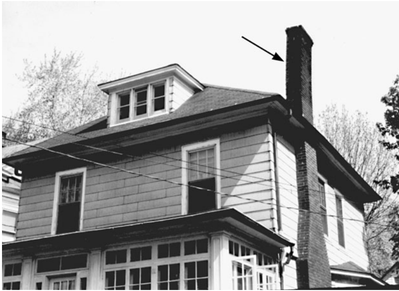
Fig. 3-3. The portion of the chimney that extends above the roof is leaning, a potentially hazardous condition.
