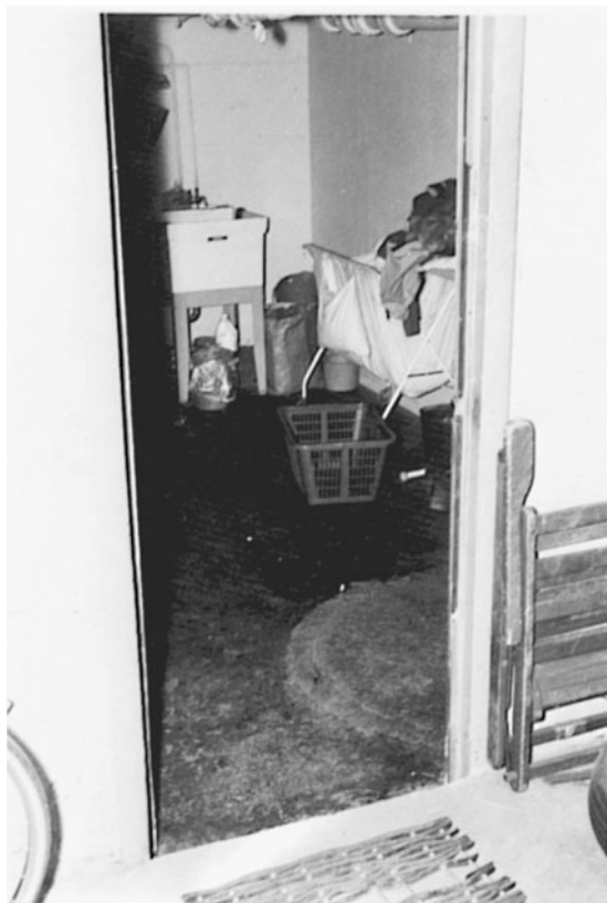
Fig. 7-2. Garage floor slab at a higher level than the adjacent living area—a potential hazard.
