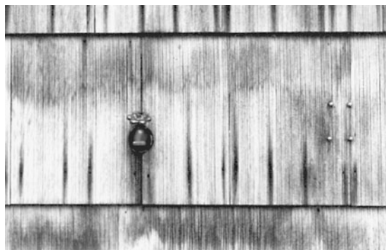
Fig. 5-2. Discolorations of wood shingles caused by rust stains from iron nails.
