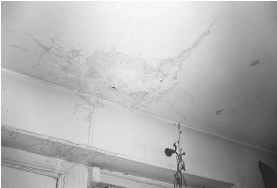
Fig. 10-8. Water stains on ceilings caused by leaks from radiator in room above.
