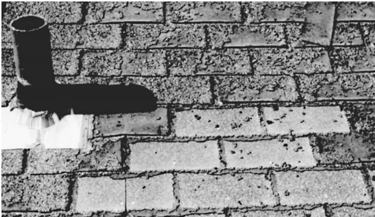
Fig. 2-5. Deteriorating asphalt roof shingles. Note torn, missing, and brittle shingles with a loss of the granule covering, exposing the roofing mat.
