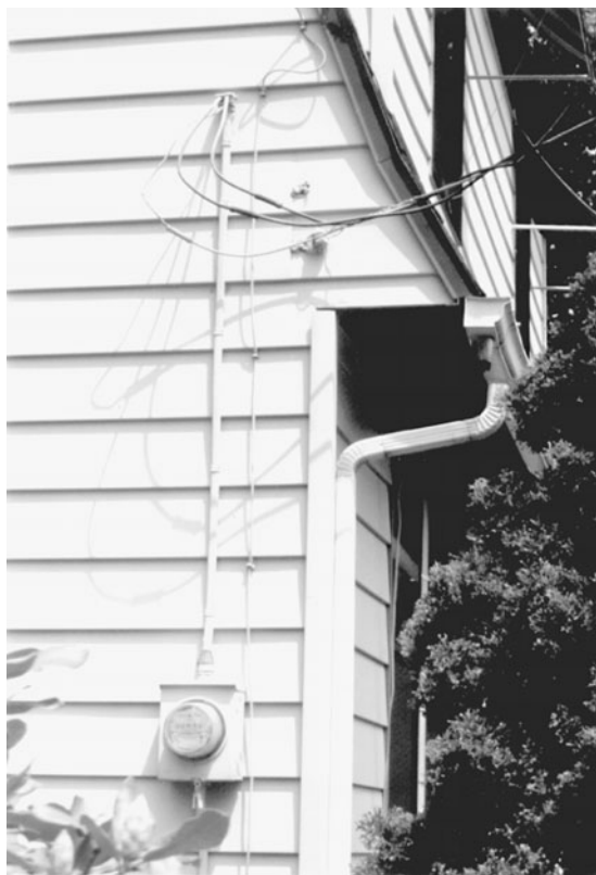
Fig. 12-2. Three-wire inlet service provides 110/220 volts.
