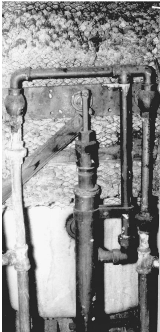
Fig. 13-8. Mixed plumbing as seen from a hallway wall hatch. Some of the fittings are deteriorating (note the rust and mineral deposits).
