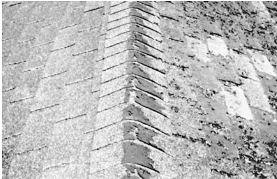
Fig. 2-2. The orientation of the house can affect the projected life of the roof shingles. The deteriorated shingles on the right slope have a southerly exposure, while the shingles on the left slope have a northerly exposure.
