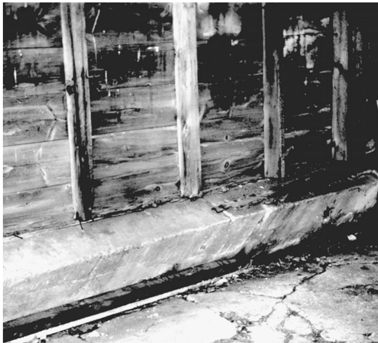
Fig. 7-9. Heaving garage wall. Section of wall was located below grade level.
