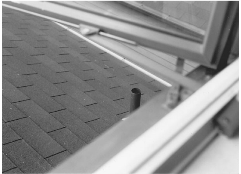
Fig. 3-9. Plumbing vent stack terminating near window. If the window is open, the discharging sewer gases can be blown into the house.
