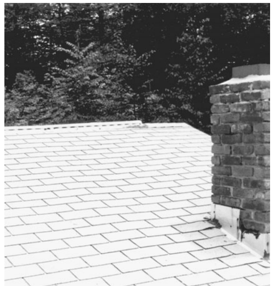
Fig. 2-1. Ridge vent. Note the ridge vent along the top of the roof. This low-profile ventilator helps circulate air through the area below the roof deck.
