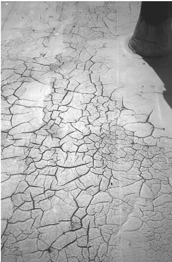
Fig. 2-11. Roof surface with alligator-type cracks.
