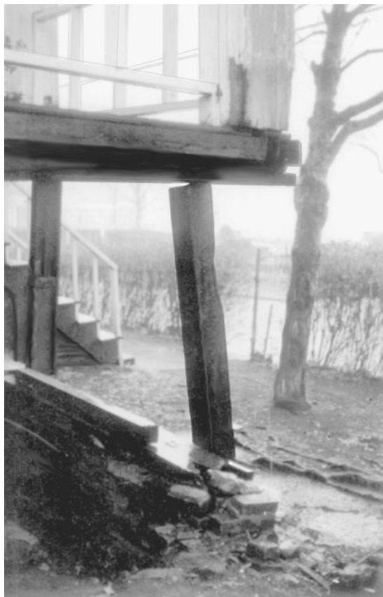
Fig. 6-18. Inadequately supported deck. Column is loose and can easily be knocked over.
