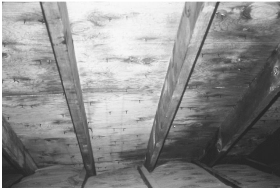
Fig. 9-8. Mildew on underside of roofing deck.
