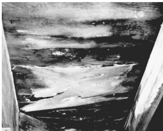
Fig. 9-9. Delamination of roof sheathing resulting from inadequate ventilation of attic.
