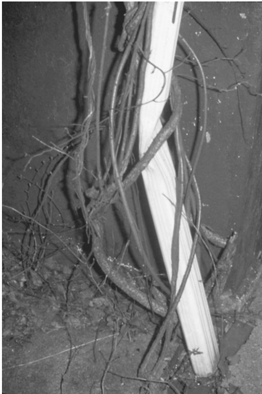
Fig. 6-16. Downspout crushed by vines.
