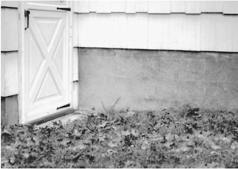
Fig. 6-6. Improper grading of the land adjacent to the house. The lawn pitches toward the door, resulting in surface water ponding in front of the entry area.
