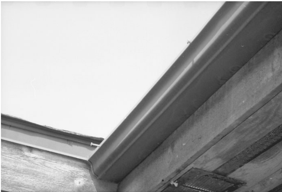
Fig. 3-11. Loose gutter spike. Should be reset and resecured.
