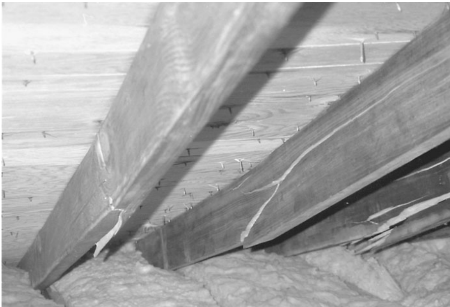
Fig. 9-11. Cracked and broken roof rafters.
