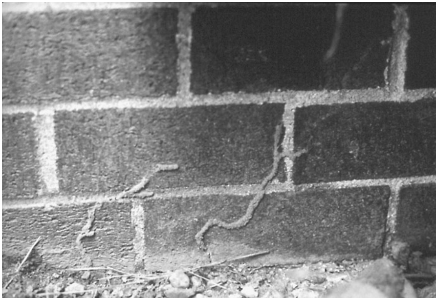
Fig. 8-6. Termite shelter tubes at base of exterior wall.
