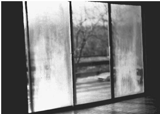
Fig. 10-6. Faulty seal in thermal-pane windows adjacent to a sliding glass door. Restricted visibility is caused by condensation between the glass panes.
