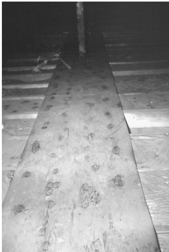
Fig. 9-7. Water-droplet stains on catwalk in attic due to condensation on protruding roofing nails because of inadequate attic ventilation.
