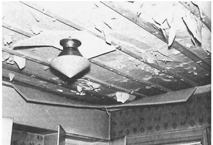
Fig. 10-2. Ceiling that had been covered with tiles, which came loose and fell down. Note that the tiles had been installed to cover a cracked, broken, and peeling ceiling.
