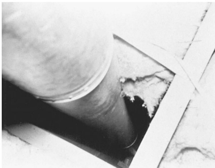
Fig. 9-4. Open joint between chimney and attic floor—a potential fire hazard.
