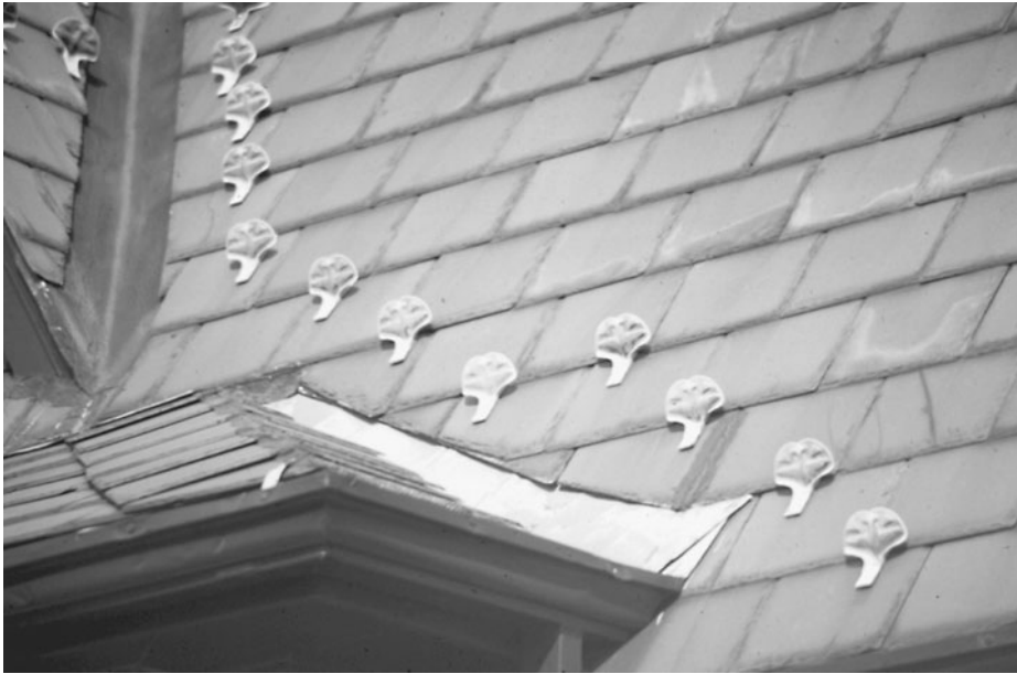
Fig. 2-9. Snow guards along the edge of the roof will help keep the snow from sliding off.
