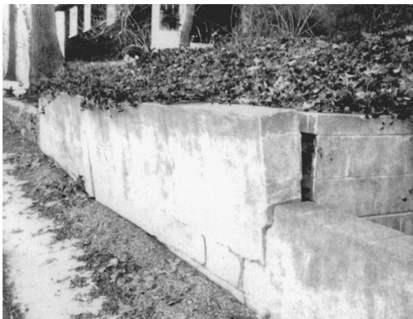
Fig. 6-13. Cracked and heaved retaining wall.
