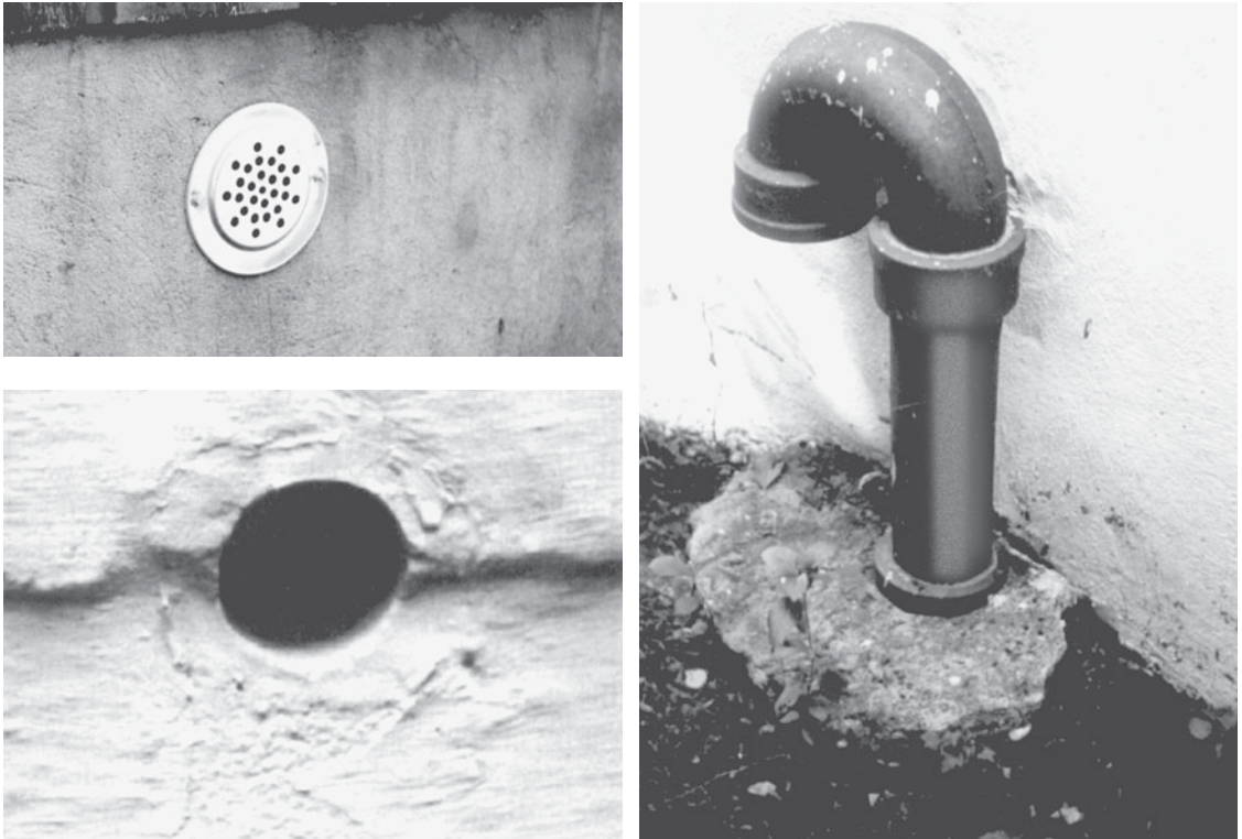
Fig. 13-3. Terminations of fresh air vent: top left—perforated plate covers opening in foundation wall; bottom left—perforated cover plate for vent opening is missing, a common condition; right—a freestanding “gooseneck” cover.
