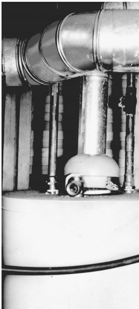
Fig. 16-2. If this relief valve discharges, someone standing nearby could be scalded. The relief valve should have an extension that discharges into a bucket located on the floor.
