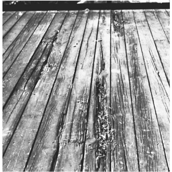
Fig. 6-20. Cracked and rotting deck planks. Planks should be replaced as needed.
