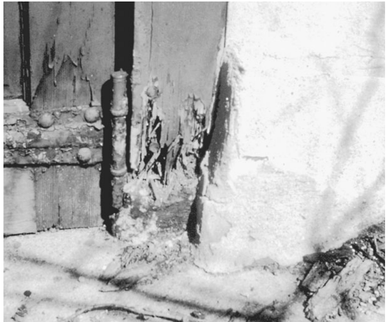
Fig. 7-8. Termite infestation and rot at base of garage door frame.
