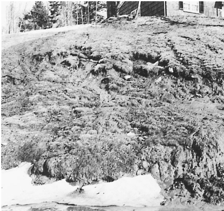
Fig. 6-2. Bank erosion on a steep slope. Correcting this condition will require a retaining wall with adequate drainage.
