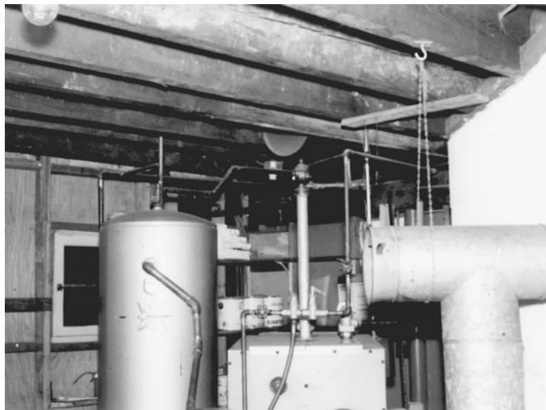
Fig. 11-13. Exposed wood joists above heating-system boiler—a potential fire hazard—should be covered with fire-code plasterboard.
