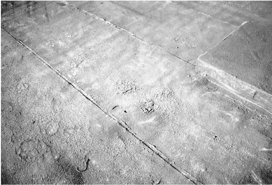
Fig. 2-12. Weathered, cracked, and aging roof membrane.
