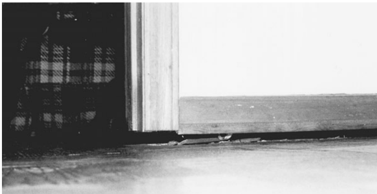
Fig. 10-3. Settled concrete floor slab. Note open joint between floor and partition walls.
