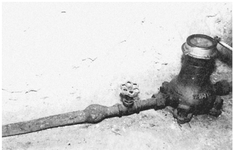
Fig. 13-9. Lead inlet water pipe. Note wiped joint (bulge) near shutoff valve.
