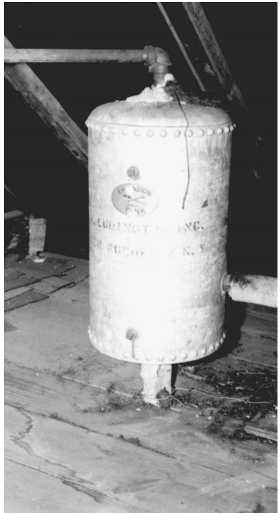
Fig. 14-6. Expansion tank for “open” gravity hotwater system—located in attic.
