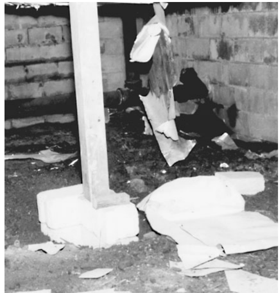
Fig. 11-17. Loose, hanging insulation in crawl space.
