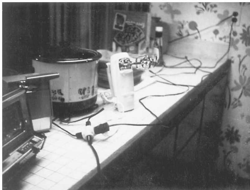
Fig. 12-9. The home wiring “octopus”—a potential fire hazard.
