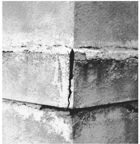
Fig. 5-5. Cracked stucco wall. If wall was covered with vines, these cracks would be concealed.
