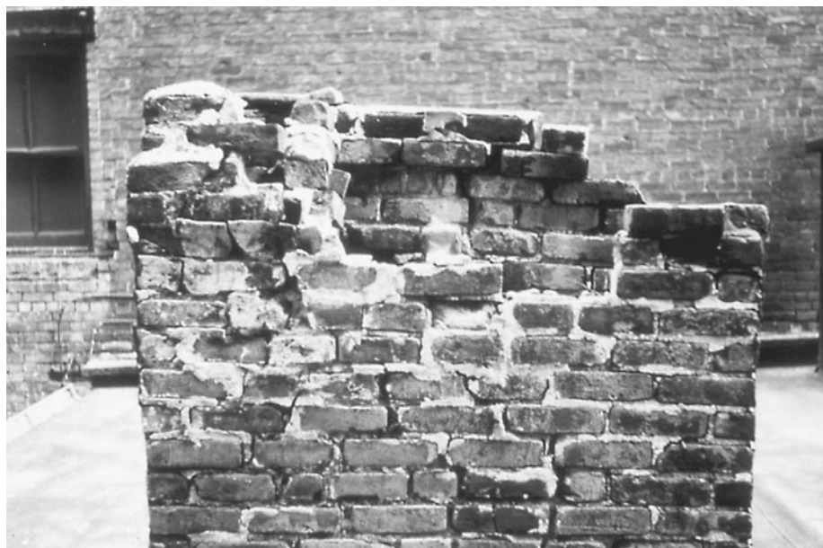
Fig. 3-5. Deteriorated chimney with no flue liner. Chimney should be rebuilt and flue should be lined.
