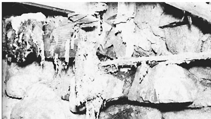
Fig. 11-15. Cracked and rotting wood-frame members in crawl space.
