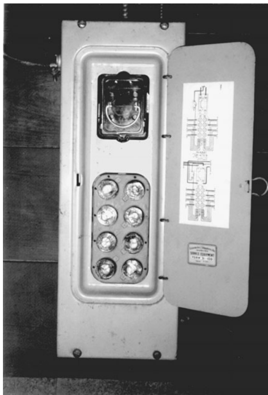
Fig. 12-5. Fuse panel box with master disconnect.
