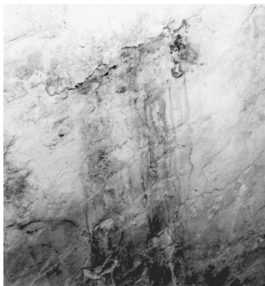
Fig. 11-9. Efflorescence and water stains on foundation wall.
