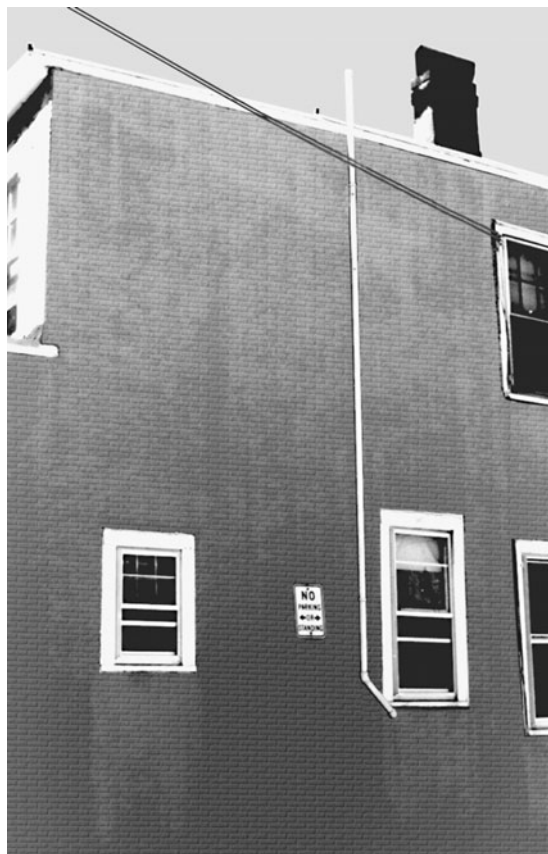
Fig. 3-8. Exterior-mounted plumbing vent stack.
