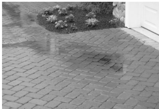
Fig. 4-6. Water ponding on a paving block driveway.
