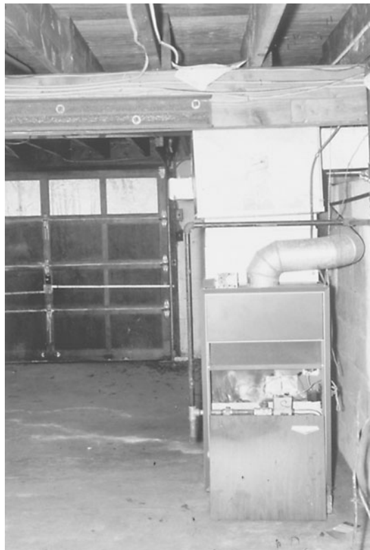
Fig. 7-4. Furnace located in the garage. Note that the ceiling should have been covered with fire-rated gypsum board.
