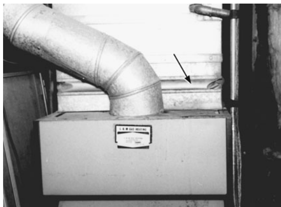
Fig. 14-3. Canvas fabric cover over the separation between the furnace and the main duct. The separation isolates the distribution system from noises and vibrations that may develop in the furnace.
