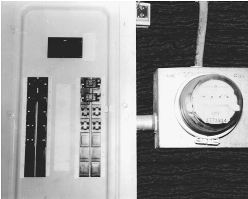
Fig. 12-4. Circuit-breaker panel box with master disconnect.
