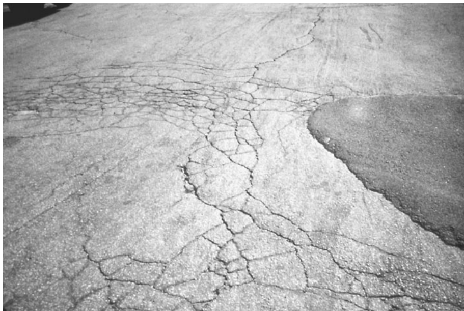
Fig. 4-5. Extensively cracked and deteriorating driveway.
