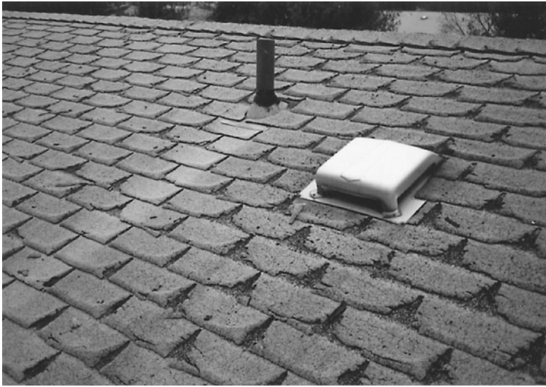
Fig. 2-7. These old, weathered asphalt roof shingles are dry, brittle, cracked, chipped, and excessively curled.
