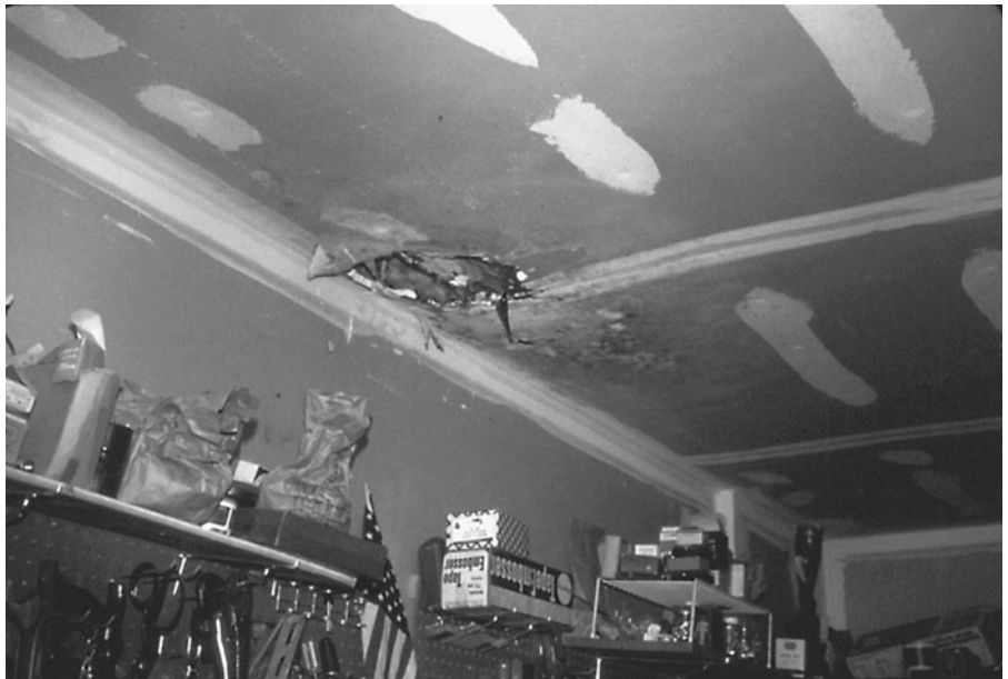
Fig. 7-6. Plumbing leak caused water-damaged ceiling in garage.
