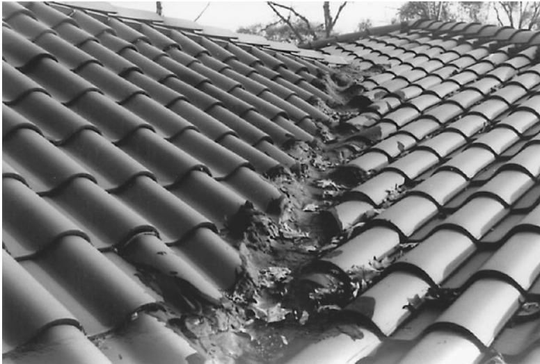
Fig. 2-10. Valley joint filled with a heavy layer of asphalt cement is an indication of a problem condition.
