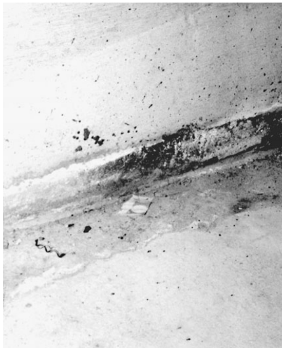
Fig. 11-10. Signs of water seepage at joint between floor slab and foundation wall.
