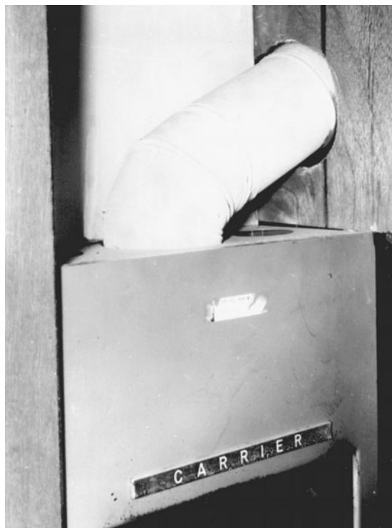
Fig. 11-14. Wood paneling near furnace—a potential fire hazard.
