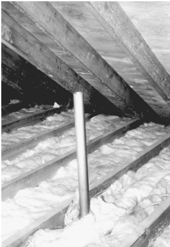
Fig. 9-1. The proper installation of insulation in the attic, between the floor joists and not the roof rafters. Note plumbing vent stack terminating in the attic—a violation of the plumbing code.
