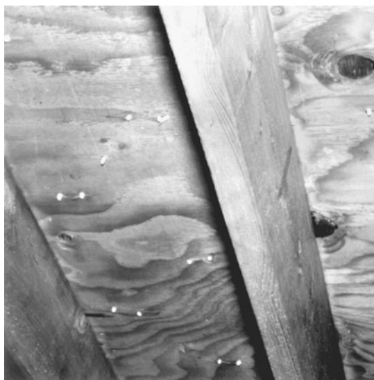
Fig. 9-6. Frost on roofing nails due to inadequate attic ventilation.
