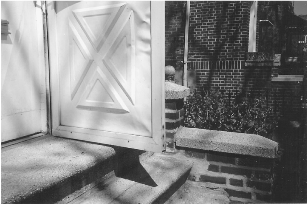
Fig. 4-4. The turnaround area of the top step is too narrow to operate the door safely.
