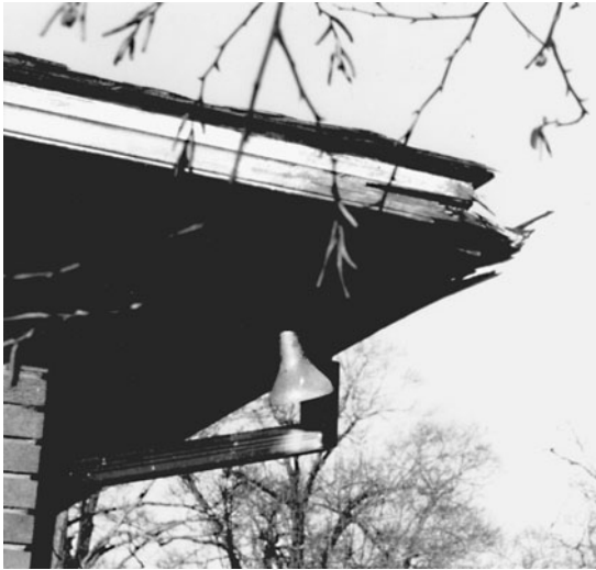
Fig. 3-10. Wood gutters. Note the cracked and rotting corner joint.
