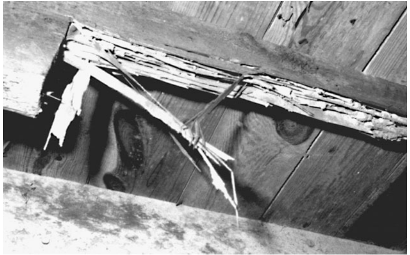
Fig. 8-7. Termite-damaged wood. Note galleries that run parallel with the grain.
