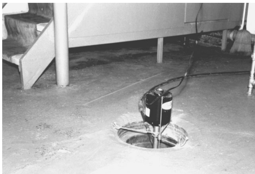
Fig. 11-12. Sump pit in center of basement floor—a tripping hazard.
