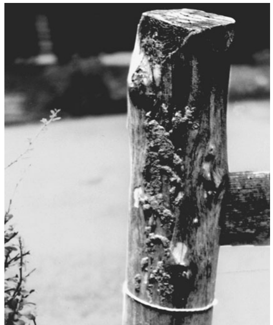
Fig. 8-8. Termite shelter tubes on a fence post.
