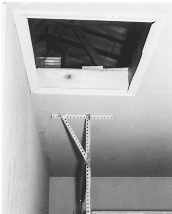
Fig. 7-3. Open attic-access hatch in the garage ceiling.
