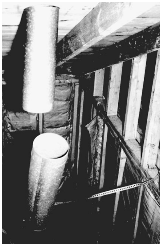
Fig. 9-3. Open joint in duct from kitchen exhaust fan.
