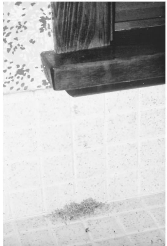
Fig. 8-10. Sawdust is an indication of carpenter ant activity in window trim.
