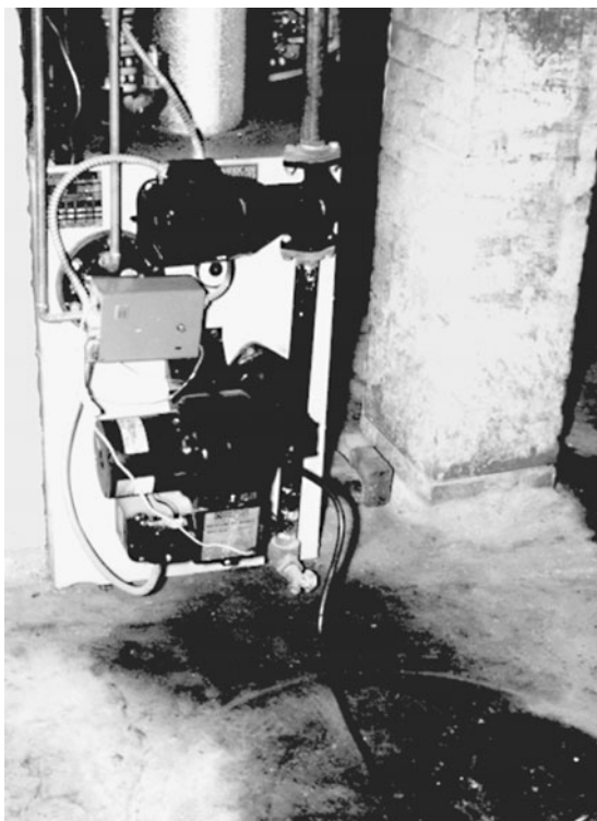
Fig. 15-1. Oil-fired forced-hot-water boiler with an exposed oil-feed line. The feed line is a small-diameter copper tube that can easily be damaged. It should be protected. Usually the feed line is located below the floor slab and emerges near the oil burner.
