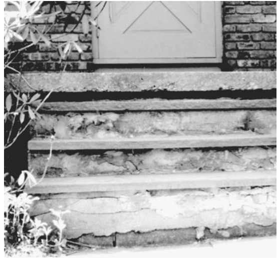
Fig. 4-3. Note that the vertical distances between the steps vary. These steps are a potential tripping hazard. The bottom riser needs masonry repair.
