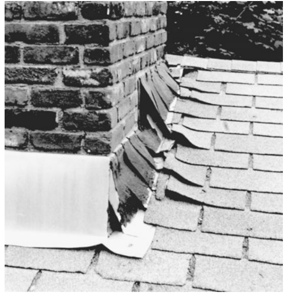
Fig. 3-2. Open and loose sections of flashing caused by movement of the chimney.
